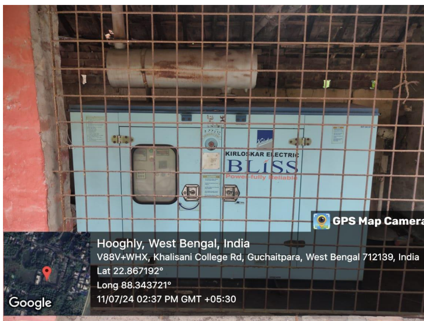
Picture 3: Diesel Generator in College Campus
